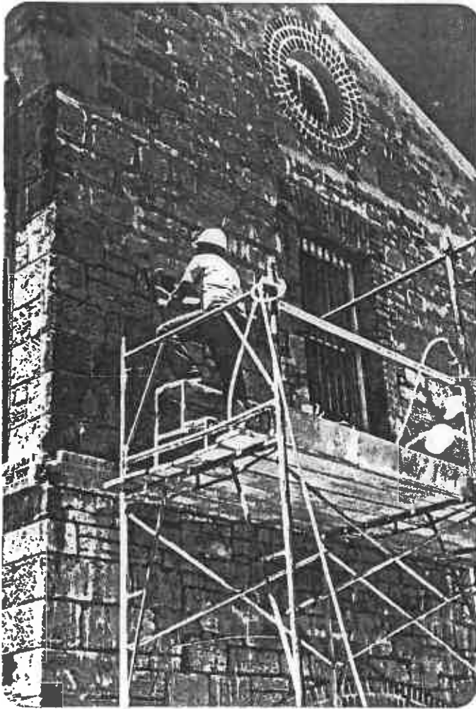
Restoration of external limestone walls by chipping and brushing - later abandoned in favour of hydrocleaning.
